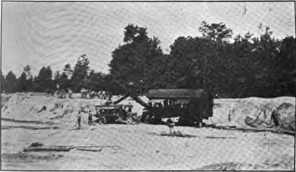
A. Working, steam shovel, and motor truck of Trent River Marl and Lime Company (Photo E. W. B.)
